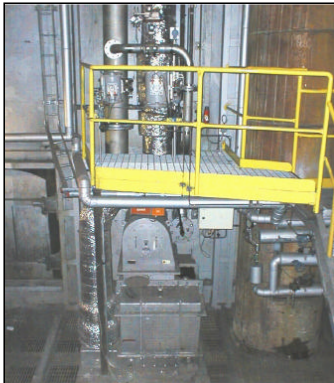
Fig. 2. Regenerative burner installation at SSAB (north side)
